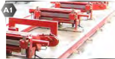
mounted in concrete
