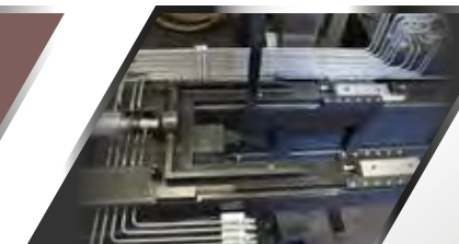
Hydraulics covered under the deck in the rails with galvanized hydraulic pipes
