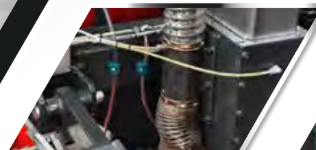
Automatic lubrication and cleaning
