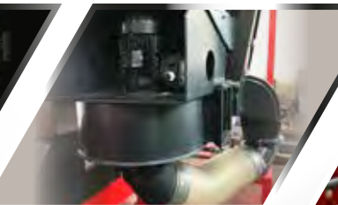
Additional sawdust exhauster system with ventilator on machine.
